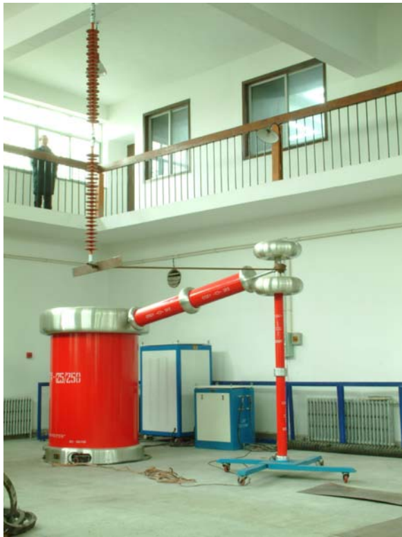
Fig. 2 The high-voltage hall on the ground floor.
