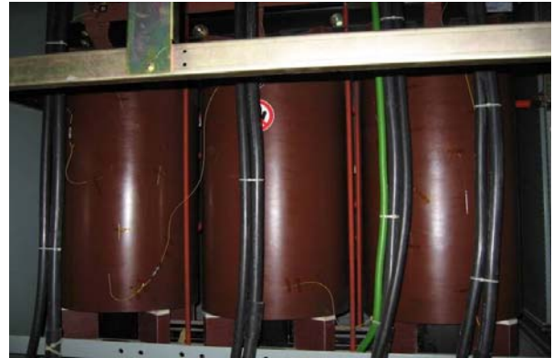
Fig. 1 The 3000kVA mold transformer with the 10 FBG sensors to monitor temperature distributions for 2 months in operation.
