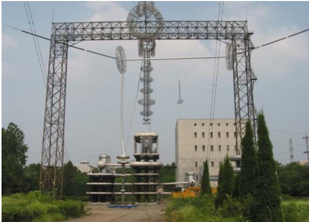
Fig.4 Outdoor test field of UHV AC Test Base, in Wuhan, Hubei province.
