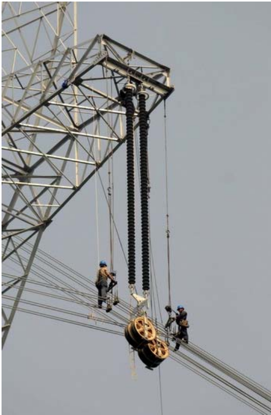
Fig.3 Under construction of the demonstration test project of AC UHV test line from Southeastern Shanxi province via Nanyang to Jingmen.
