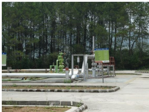
Fig. 2 Kamojang Geothermal Power Plant
