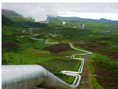
Fig. 3 Wayang Windu Geothermal Power Plant
