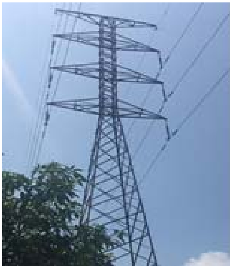
Fig. 3. Long rod type suspension insulator with operating voltage of 70 kV (30 years operation)
