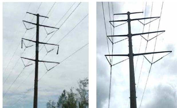
Fig. 6. 230 kV lines with polymeric insulators (24 years in operation)
