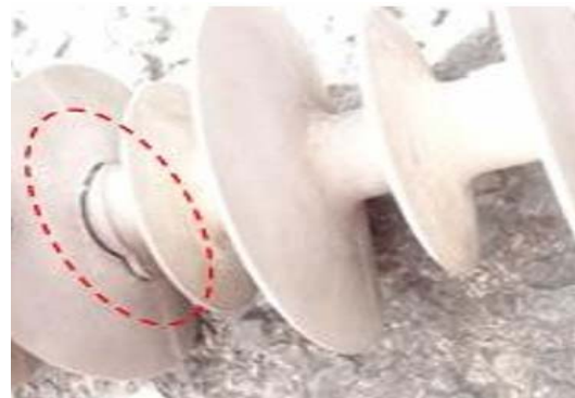
Fig. 8. 150 kV, coastal area, 5 years, corrosion of end fitting.
