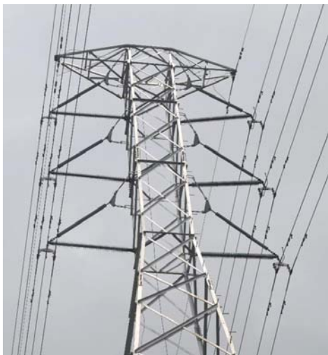
Fig. 4. Uprated tower from 70 kV to 150 kV using polymeric insulators (26 years operation)
