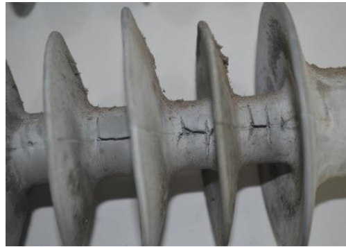
Fig. 7. Housing scratch on polymeric insulator 70 kV, 27 years operation, volcanic polluted area.
